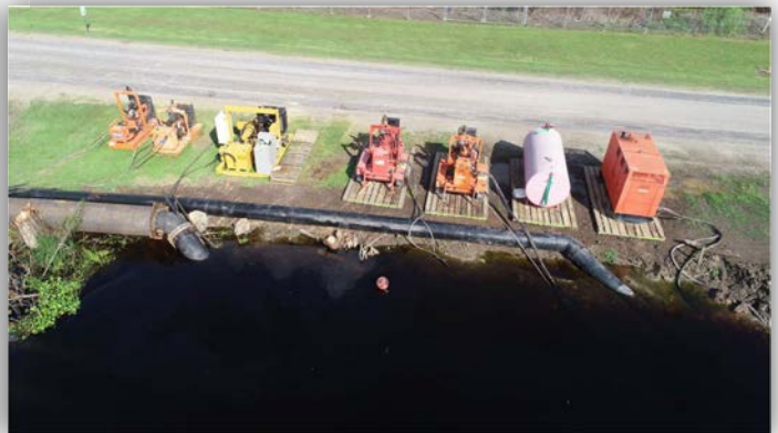
Emergency Pumps at Elliot Jones June
