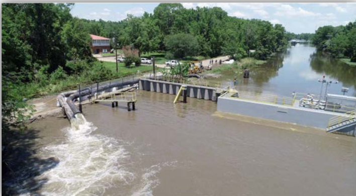
Emergency Pumps at Old Spanish Trail May 2019
